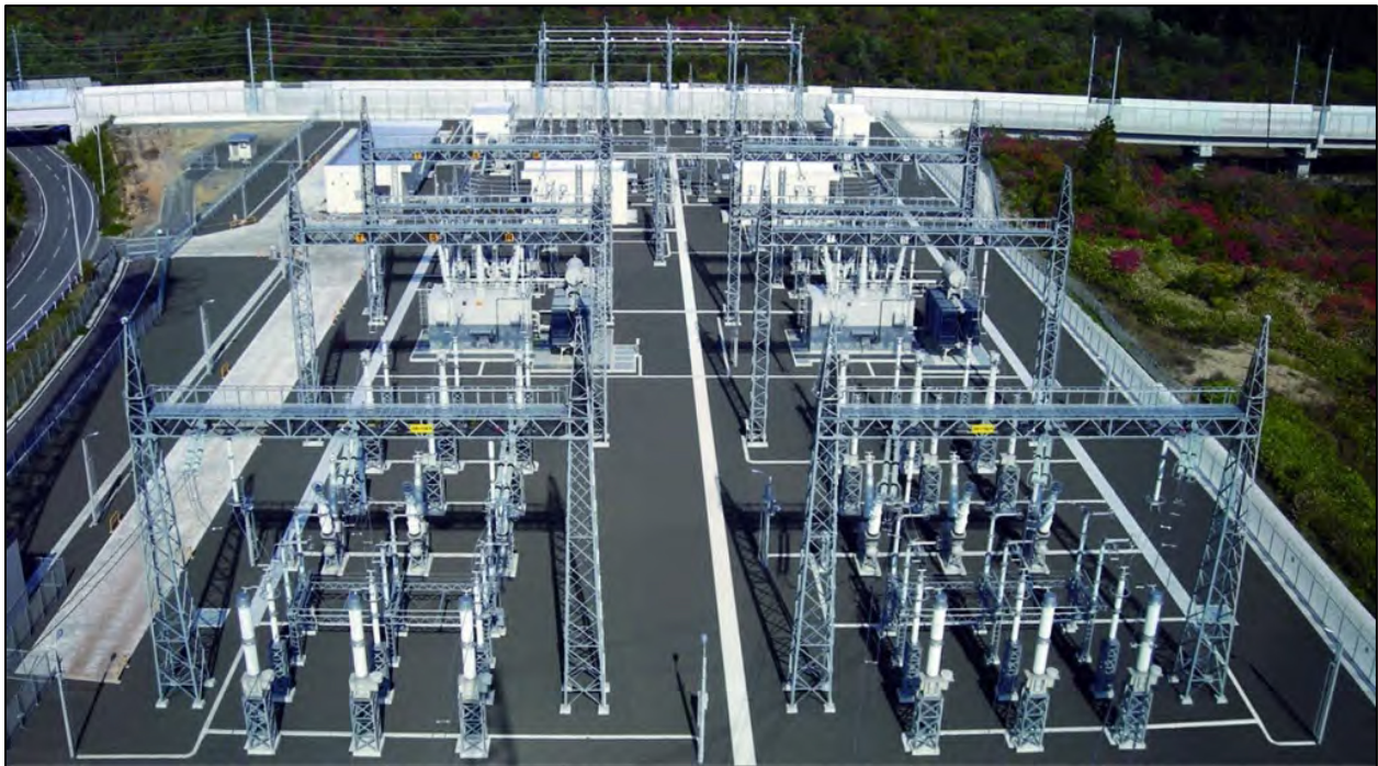
Figure 2-16: Typical HSR TPSS
