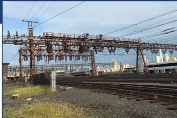
Figure 6. Catenaries may make it difficult to identify signals on signal bridges
