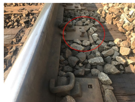
Figure 2. Uplifted spike observed in track
