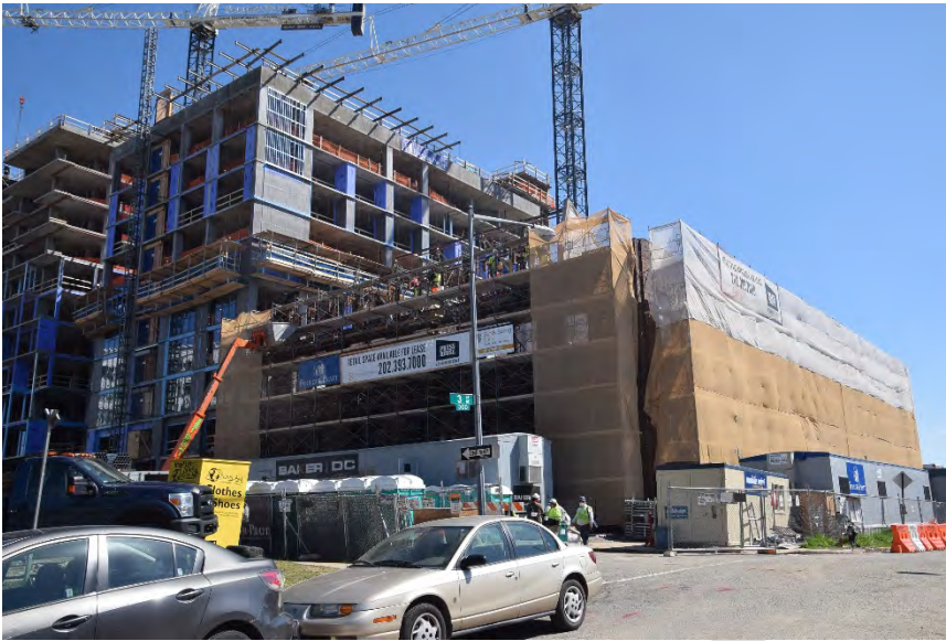
Capitol Press Building from N and Third Street NE, view looking southeast.
