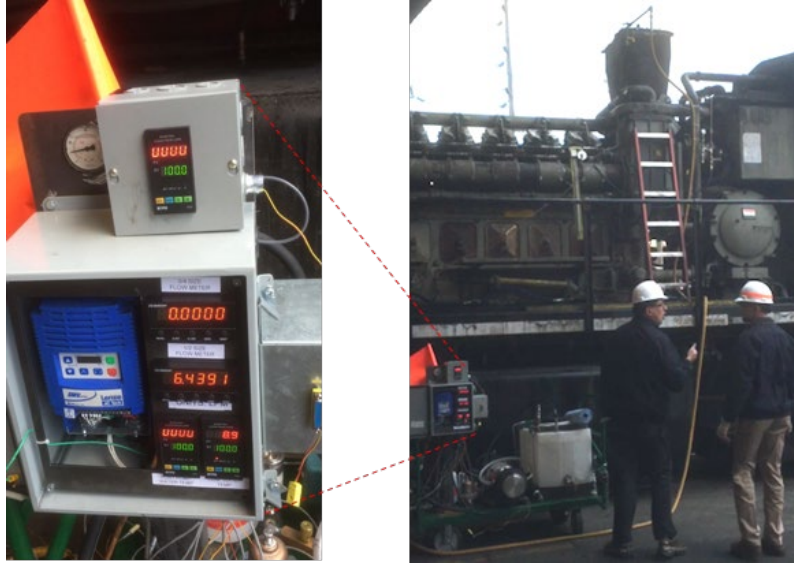
Figure 9. PDP instrumentation and connection to HiPHEX st retrofitted locomotive
