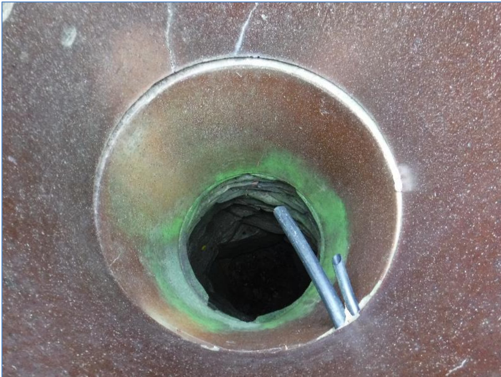
Photo 5.3-11 (Location 316) Well 2 with Metal Pipes Extending into Well Wall.
