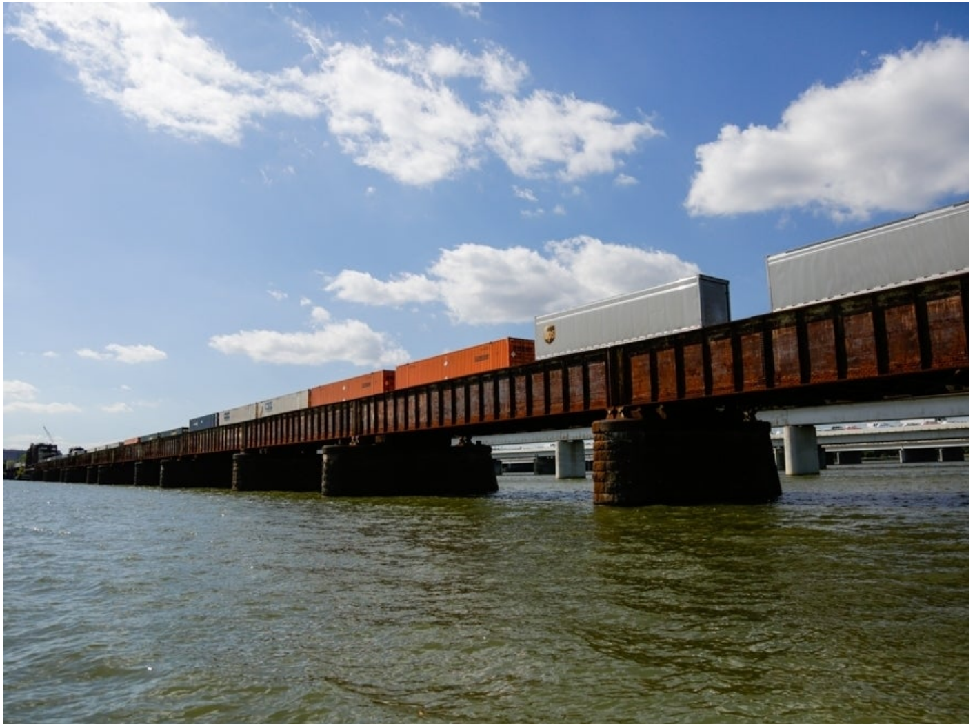
A freight train crosses the rust-covered Long Bridge over the Potomac River between Washington and northern Virginia. (Heather Kim/Capital News Service)
