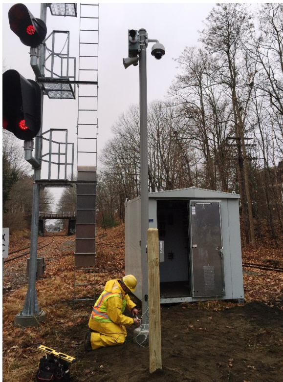
Figure 4 – Rock Junction Camera Pole
