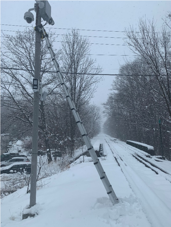
Figure 5 – Jordan Avenue Camera Pole
