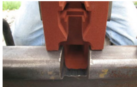
Figure 1. Thermite rail HRW process showing a portion of head removed with the mold fitted to the rail and positioned above the cutout
