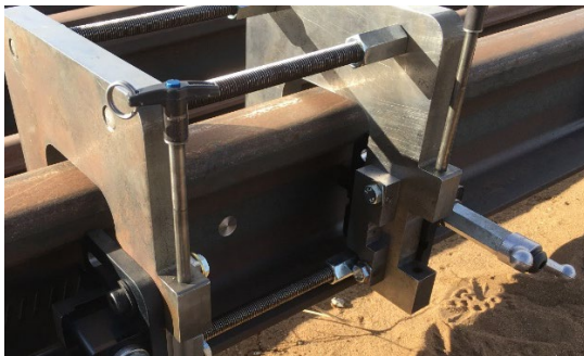
Figure 4. Rail web prepared for signal stud attachment (machined circle in center of image)
