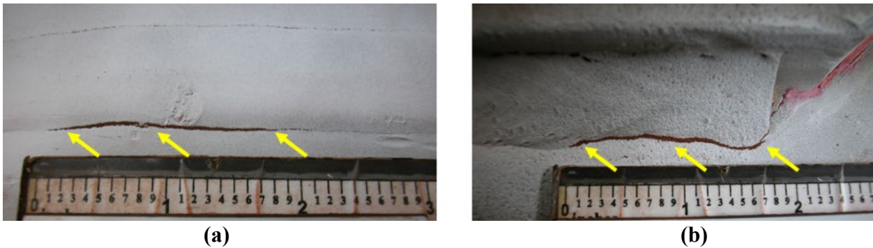
Figure 3. Contrast MT Revealing Toe Cracking in Welds; (a) BW, (b) FW
