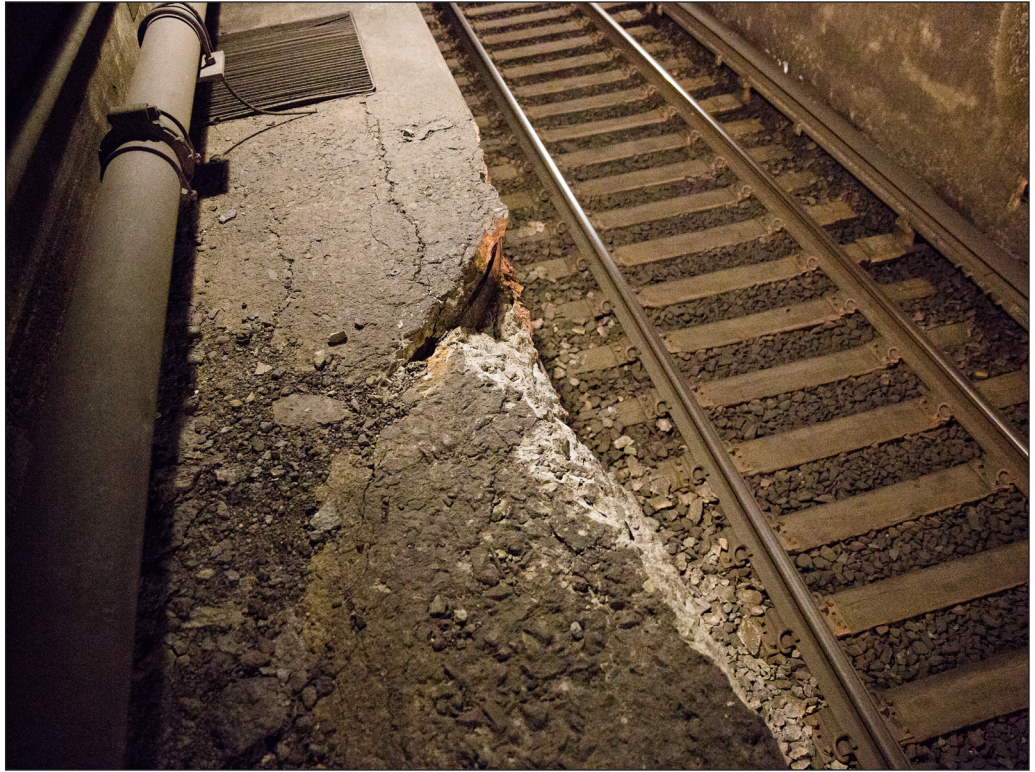
Damage to bench walls in North River Tunnel
