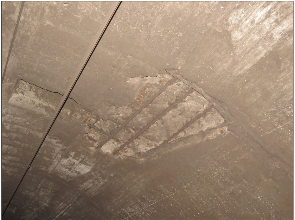
North River Tunnel damage, concrete lining
