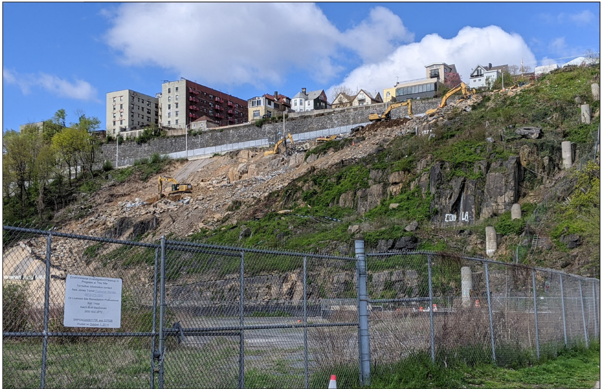
Hoboken fan plant site from West 18th Street in Weehawken, facing west 8
