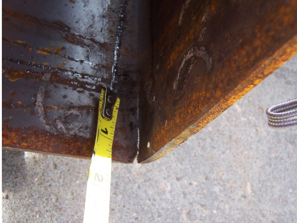
Figure 14. Photograph of cracked buffer beam channel that was rejected and re-fabricated
