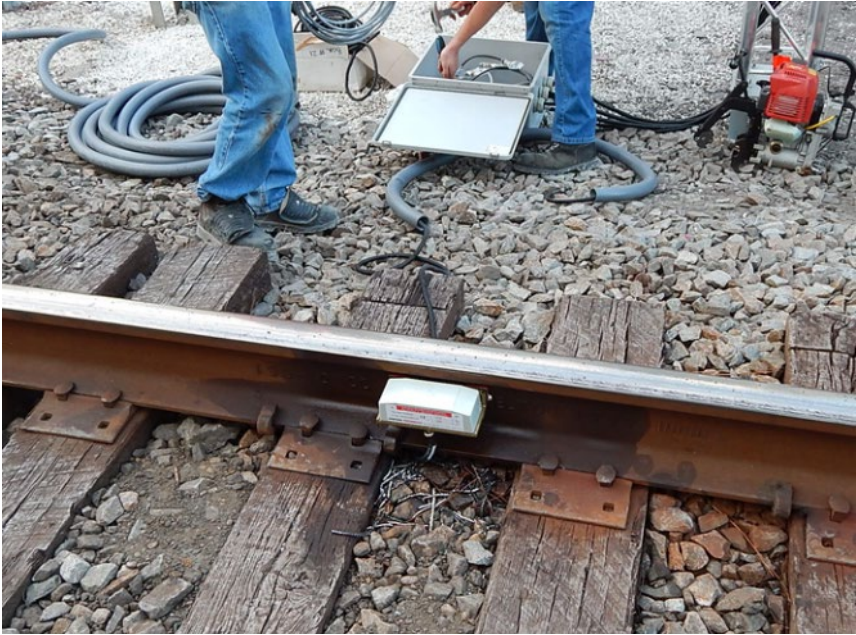
Figure 8. Wheel Sensors Mounted on Each Rail for Precise Triggering of Cameras
