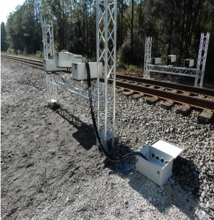
Figure 7. Nearly Completed System Showing All Cameras in Position
