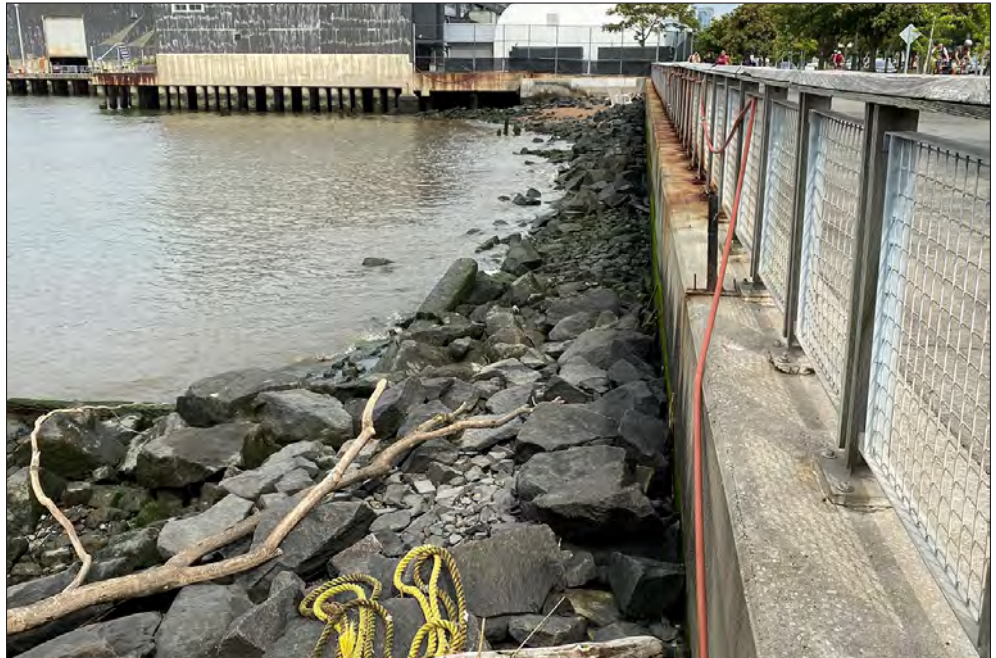
Hudson River Bulkhead, view north at Hudson River and West 34th Street 5
