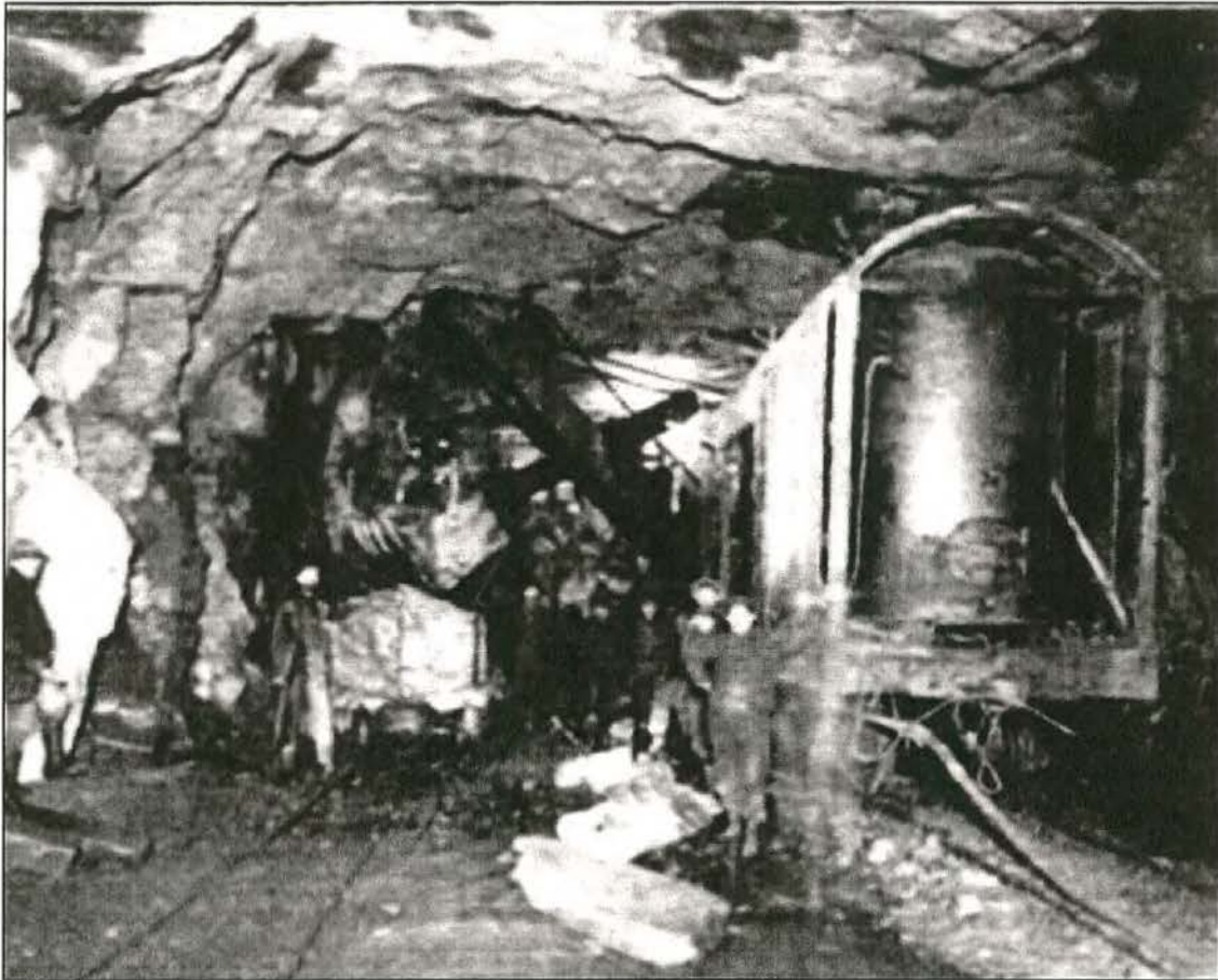
Figure 16 Air Operated Steam Shovel Used in Cross-Town Tunnel (The New York Tunnel Extension: Description of the Work and Facilities Vol. II, No.1158, Plate LIX, Fig. 1.)
