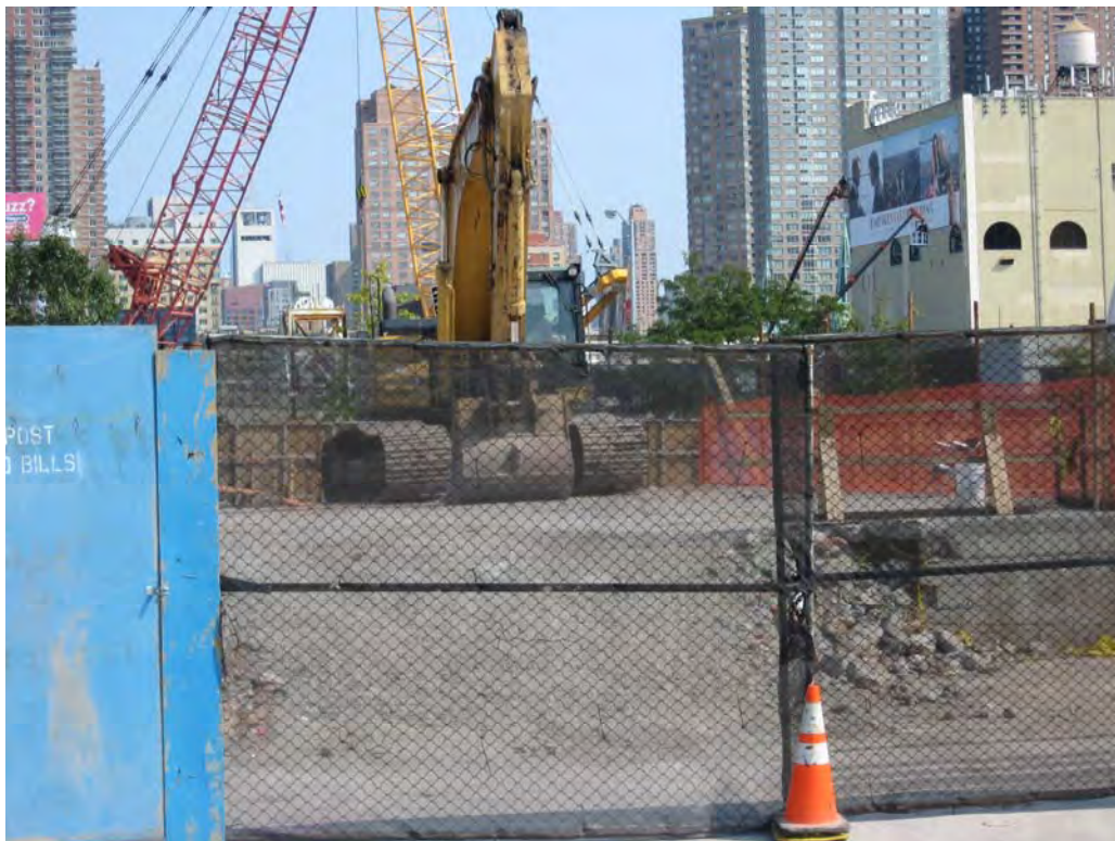
Picture 16 – (09/22/08) – Active construction site northeast of Site, north of West 33 rd Street.
