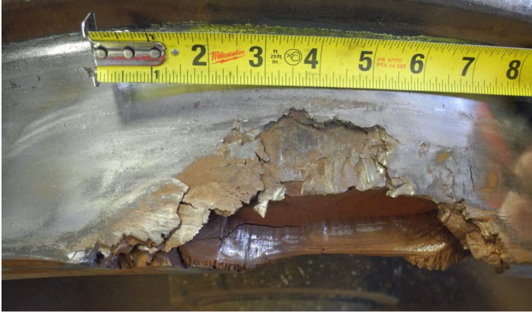
Figure A-2. Overall View of Fractured Portion
