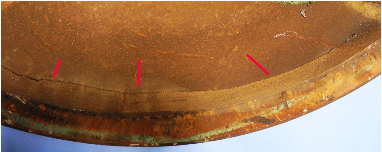
Figure A-11. Termination of VSR at Rim-Plate Fillet
