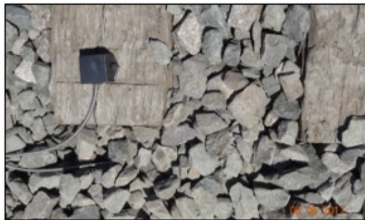
Figure 38. Accelerometer Attached to a Tie and Covered with a Plastic Box
