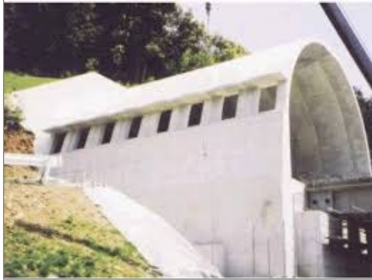
Figure 50: Type of Tunnel Hood
