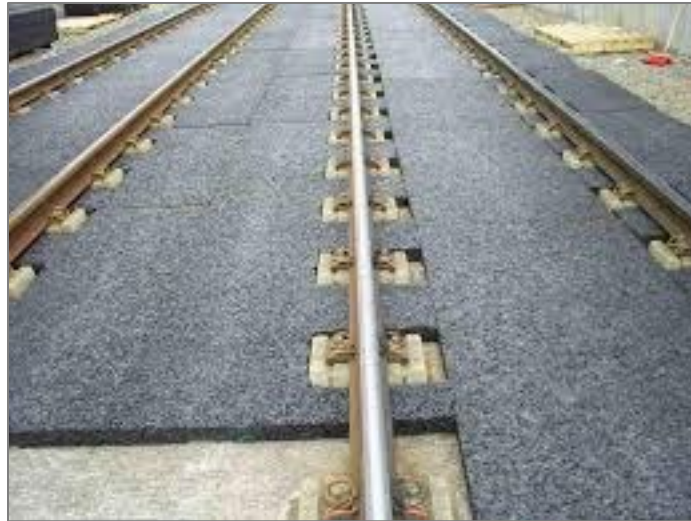
Figure 51: Damping Material Above Slab Tracks
