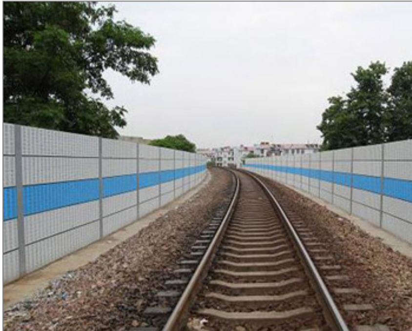
Figure 49: Sound Barriers at Edge of Right-of-way
