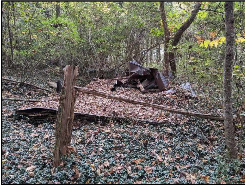
Figure 34: Collapsed Structure and Fence Posts at 31MK1173, facing Southeast
