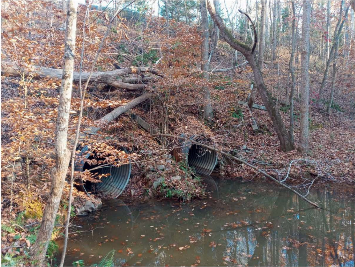
Photograph 3: View of stream S1 (b) and culverts south of existing rail line in the central portion of the site, facing northeast.
