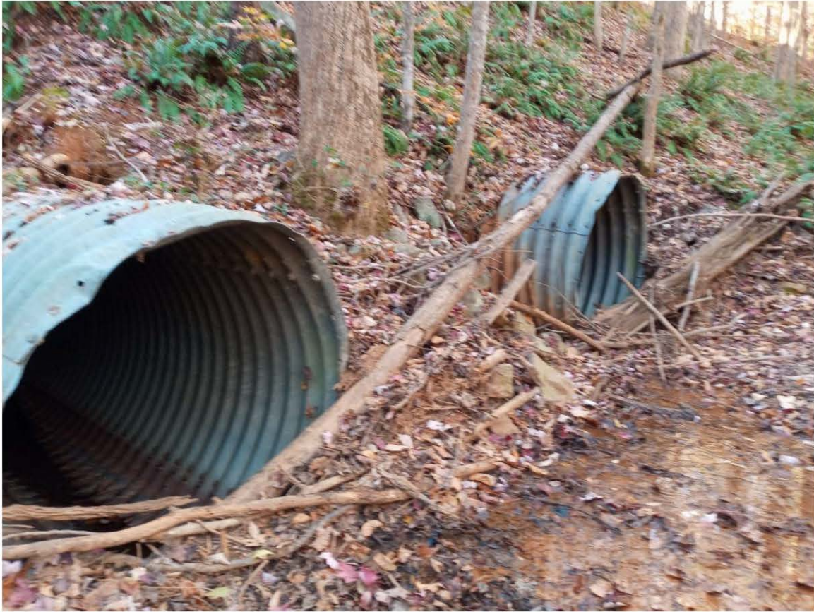
Photograph 5: View of stream S1 (a) and culverts north of existing rail line in the central portion of the site, facing west.
