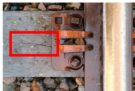
Figure 3. Tie spike-hole cracking
