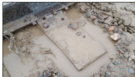
Figure 1. Photograph of track with fines and a saturated surface
