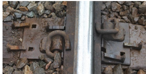
Figure 1. Broken spikes in elastic fastening system
