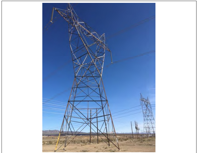
Los Angeles Department of Water and Power, Boulder Line
