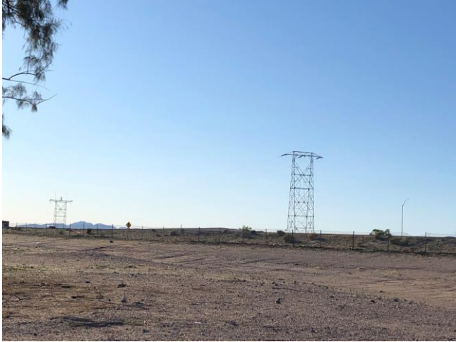
Segment 5, east end, north side. Type A dead-end tower (right), Type SW Tower (left), camera facing west
