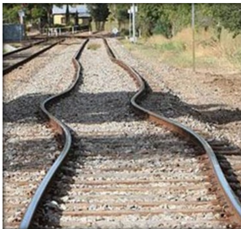
Figure 1: Photograph of a Symmetric Track Buckle
