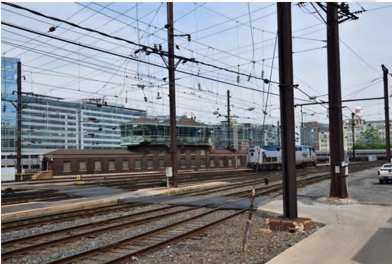
Photograph of the Terminal Rail Yard showing existing conditions of "K" Tower and several original single catenaries, looking north
