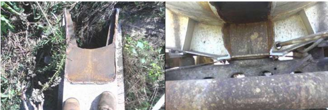
Figure 1. Stub Sill Fracture Observed in Callahan, FL, December 2009 (Sundaram, 2016)
