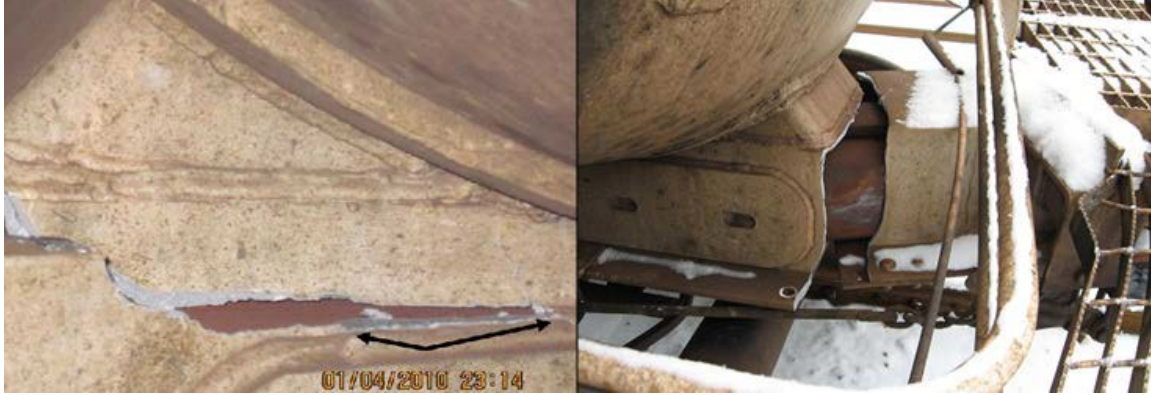
Figure 2. Stub Sill Fracture Observed in Charleston, WV, January 2010 (Sundaram, 2016)
