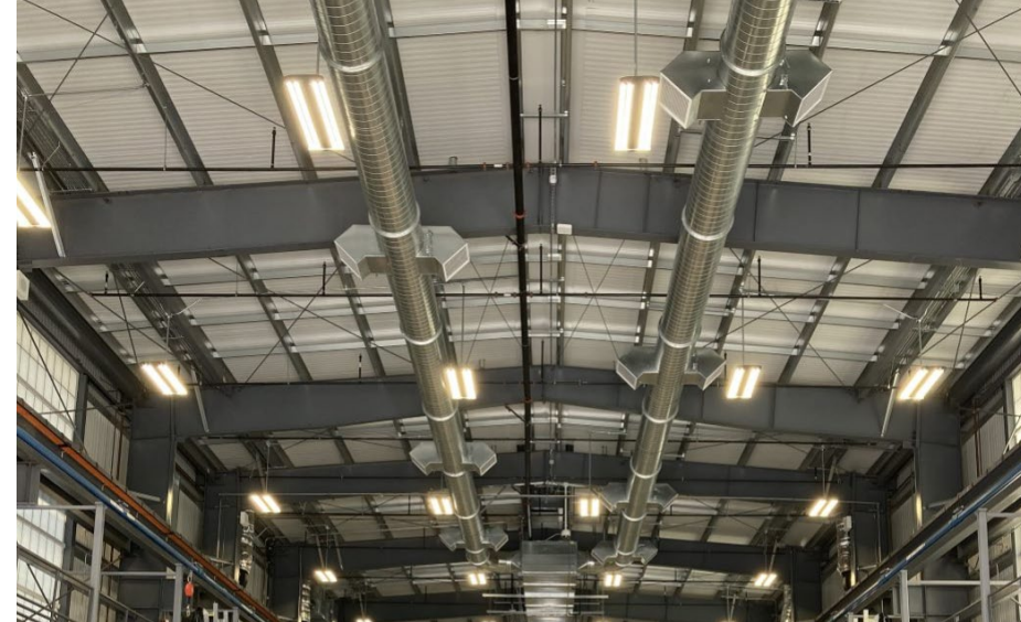
Ventilation system [Source: Mott MacDonald]
