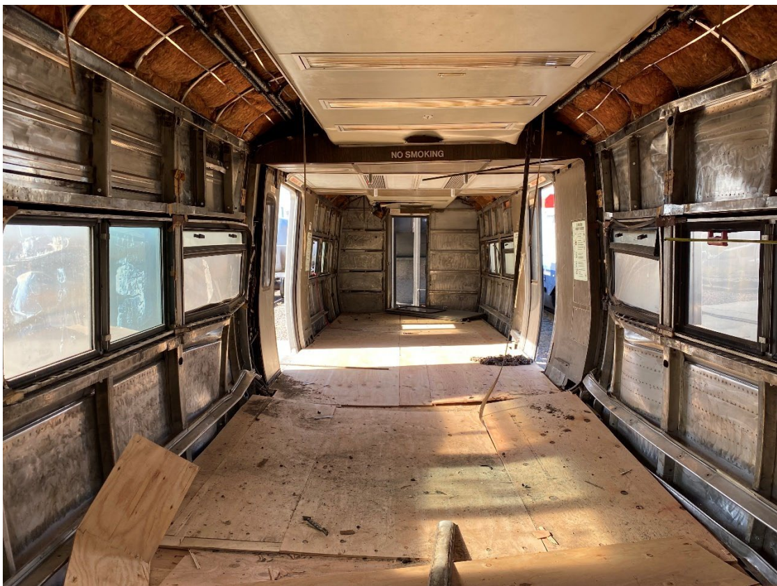
Figure 83. M1 interior damage, buckle at rear door
