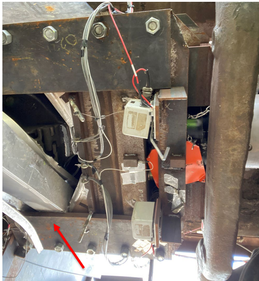
Figure 77. One of the two sliding lug support plates was deformed
