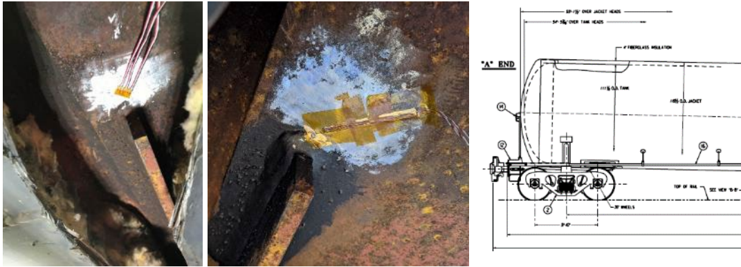
Figure 9. In-Board Strain Gage Installed Under the Car at the End of the Stub Sill Beam (Old on Left, New in Center)
