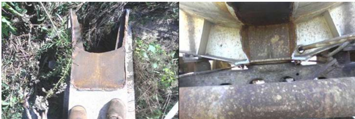
Figure 1. Stub Sill Fracture Observed in Callahan, FL, from December 2009 (Sundaram, 2014)
