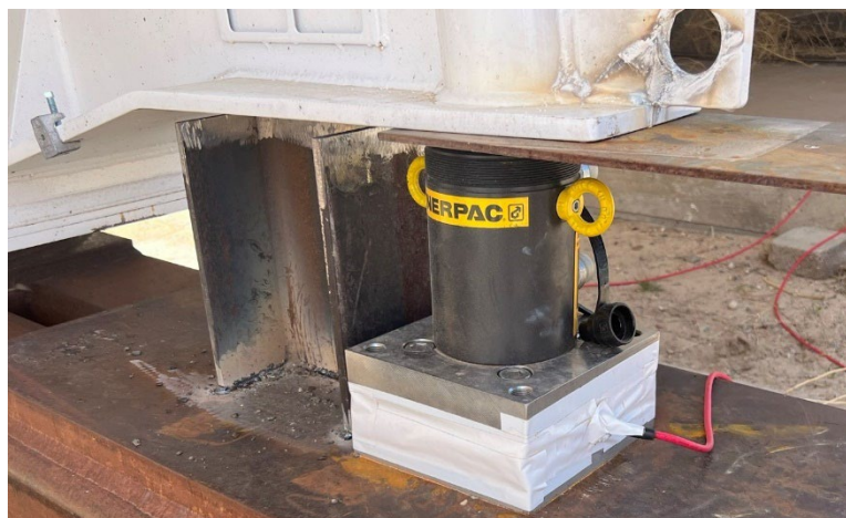
Figure 6. Load Cell with Hydraulic Ram Positioned on Top to Transfer Weight from Center Plate to Load Cell
