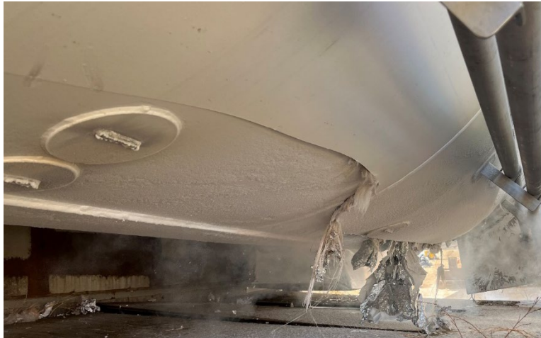
Figure 23. Split in Bottom of Tank Caused by Thermal Stress
