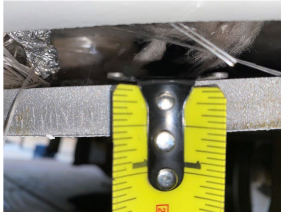
Figure 25. Thickness of Outer Tank Along Thermal Crack
