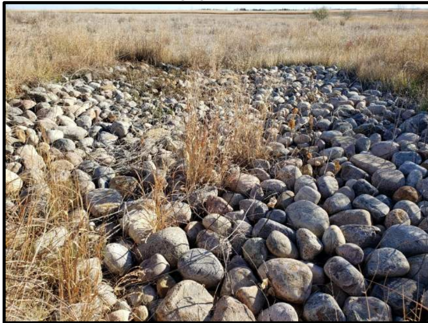
Photo 58. Direction: East. OW11 riprap erosion control apron at end of ditch.
