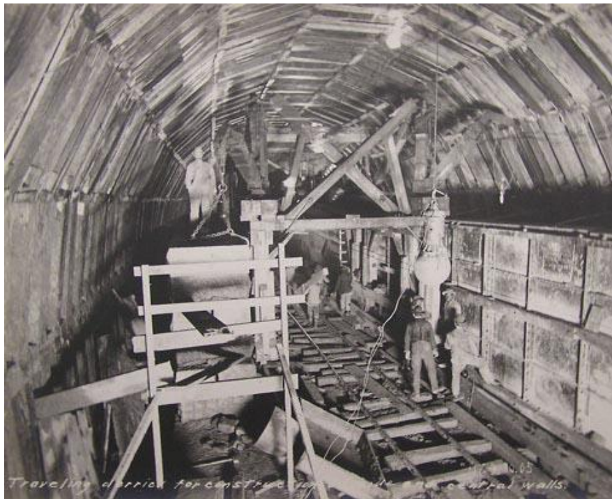
Figure 30. Crews using a traveling derrick for constructing the side and central walls of the First Street Tunnel. Source: C.K. Allen Collection. Between 1904-1905. Photograph. From the Library of Congress.
