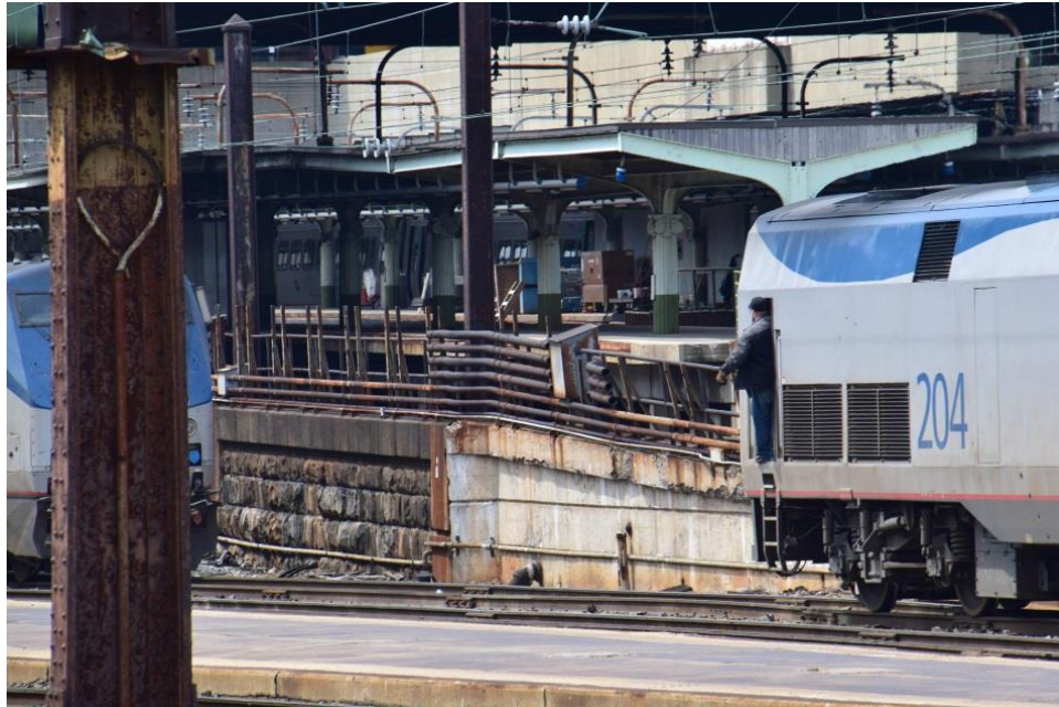
Figure 18. Photograph of Terminal Rail Yard showing the existing conditions of the platforms and umbrella sheds, looking southwest. The cast iron columns have been repainted and the roof structure modified. The stone retaining wall, dividing the high-level tracks and platforms from the lower-level tracks and platforms can be seen in the foreground. Source: BBB, 2017.
