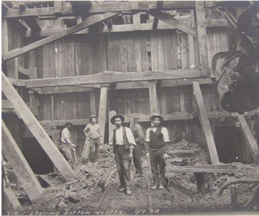
Figure 29. Crew members at the bottom of drifts during construction on the First Street Tunnel. Source: C.K. Allen Collection. Between 1904-1905. Photograph. From the Library of Congress.
