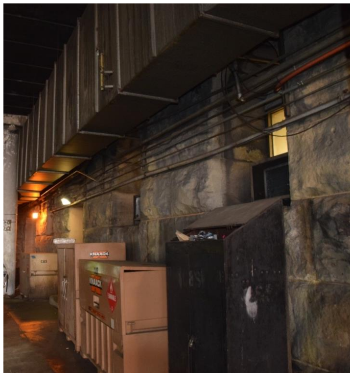
Figure 24. Looking southeast, along the First Street Tunnel beneath Union Station, featuring quarry faced Potomac stone. Source: BBB, 2017.
