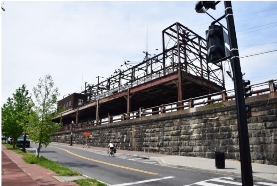
Figure 22. Photograph of the Substation 25A and eastern retaining wall below, looking southwest. Source: BBB, 2017.
