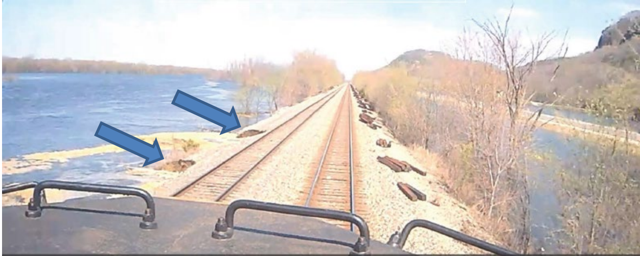
Figure 2: Photo from the rear Distributed Power Unit on Train-53 at MP 268.8. Note the two areas of erosion adjacent to Main-2 (arrows).
