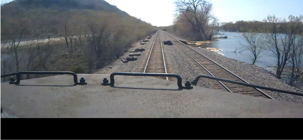
Figure 3: A photo from Train-25 locomotive camera recording shows the degradation of the track structure under Main-2 as it approaches the area of concern.
