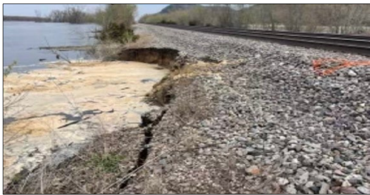
Figure 1: Photo from April 27, 2023, of the derailment area taken by RW3 who was placing stone to stabilize the bank of the river before the derailment. RW1 received the photo at approximately 10:30 am.
