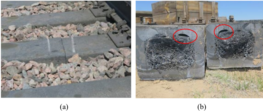
Figure 4. Center cracking observed in new EPC tie test zones: (a) Center cracking in tie type A at 120 MGT; (b) Initiation of crack at void (circled)
