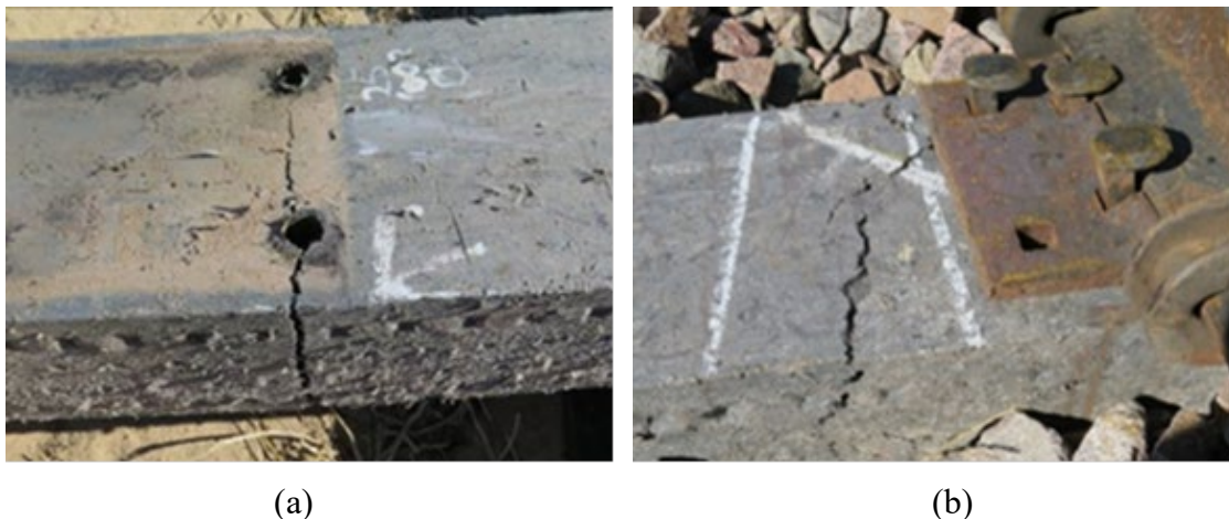
Figure 5. Spike-hole cracking observed in new EPC tie test zones: (a) Spike-hole cracking in drive spike holes of tie type B; (b) Spike-hole cracking in cut spike holes of tie type C
