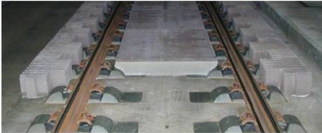
Figure 8-11. Acoustic absorbers fitted in Euerwang Tunnel, from [69], photographer Peter Deeg, DB Systemtechnik GmbH
