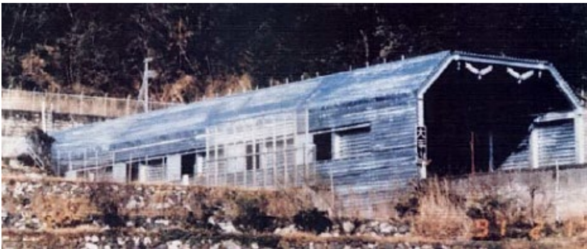
Figure 8-7. Japanese tunnel entrance hood (steel) – retro-fitted to Ohirayama tunnel, from Maeda et al [94]; reproduced by kind permission of the authors
