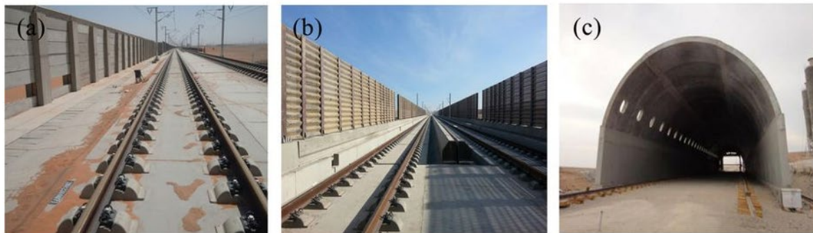
Figure 6-11. Main wind protection structures along the Lanxin Railway II [17]. (a) Subgrade wind barriers; (b) bridge wind barriers; (c) wind-proof tunnels
