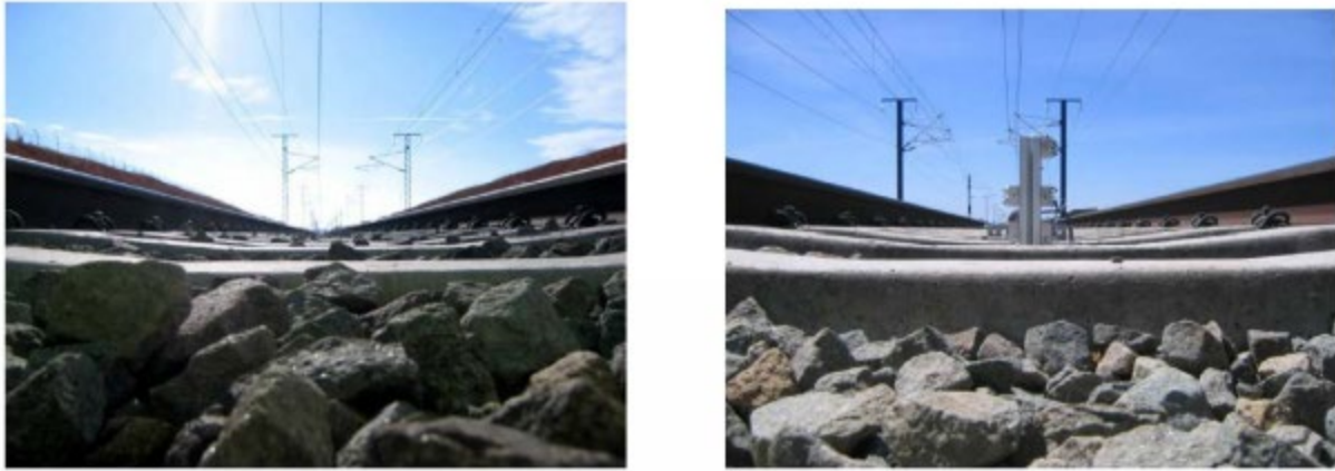
Figure 10-2. Left: Typical track ballast conditions. Right: lowered profile ballast less susceptible to aerodynamic effects from trains (Figure 3.3 from [45])
