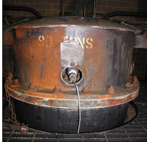
Figure 5. Pressure Transducer at Manway Longitudinal Tank Shell Strain on the Top of the Tank
