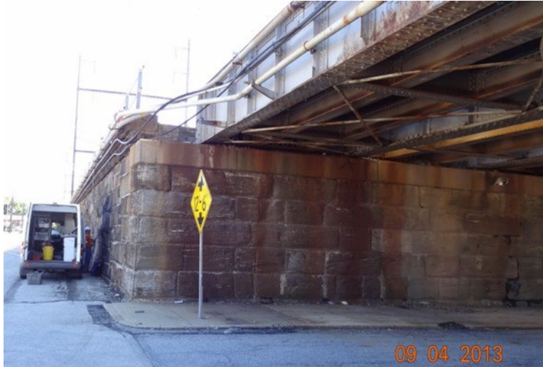
Figure 179. Masonry walls at Upland Avenue below the Upland (15 ft) instrumentation location, looking north with truck adjacent to wall with MDD location on Track 3 above the truck
