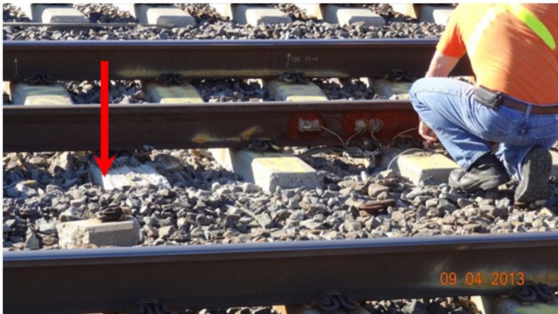
Figure 62. Damaged tie to the left of the MDD instrumentation location (see red arrow) at Madison (12 ft) on 4 September 2013
