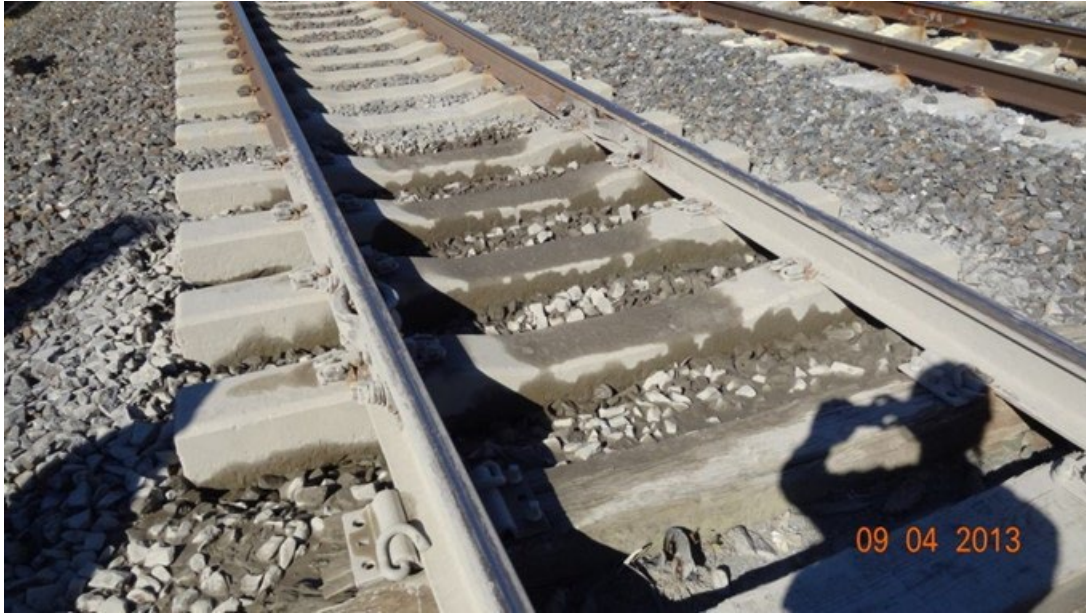
Figure 65. Fouling material covering ballast and concrete ties on Track 1 at Madison (12 ft) on 4 September 2013
