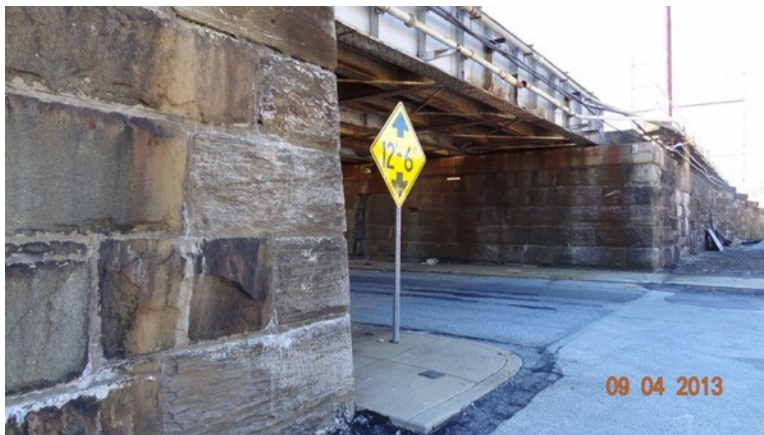
Figure 180. Masonry walls at Upland Avenue below the Upland (15 ft) instrumentation location, looking south, showing single-span bridge over Upland Avenue
