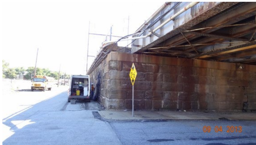
Figure 3. Photograph of masonry walls at Upland Avenue below the Upland (15 ft) MDD location
