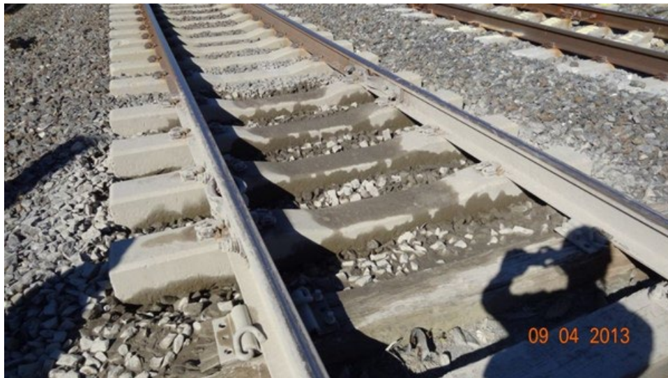
D.1. Fouling material covering ballast and concrete ties on Track 1 at Madison (12 ft) on 4 September 2013
