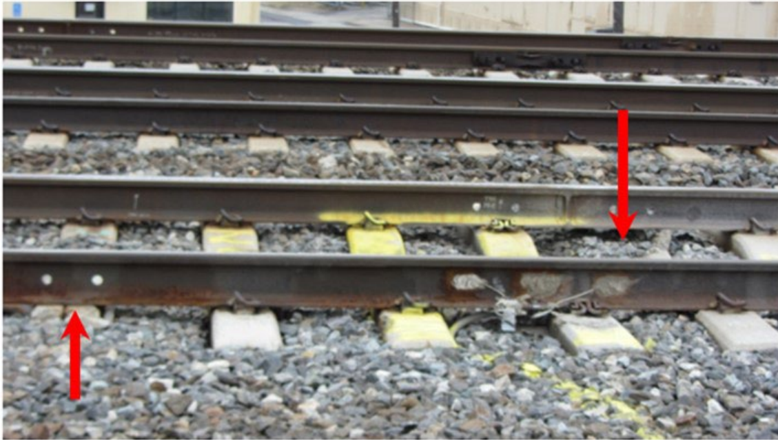
Figure 63. Photo of two damaged ties near the Upland (15 ft) instrumentation location (red arrows) (Damaged ties are three ties to the left and one tie to the right of the instrumented tie)
