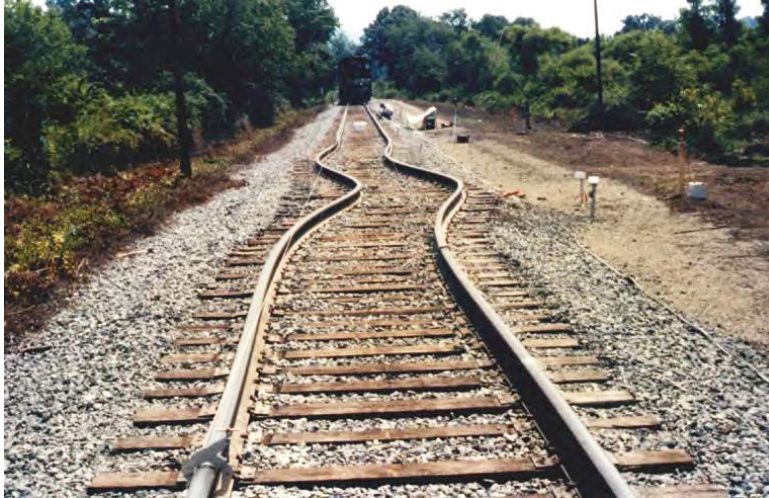
Figure 13. An example of rail buckling due to high temperatures on a track with timber rail ties.
