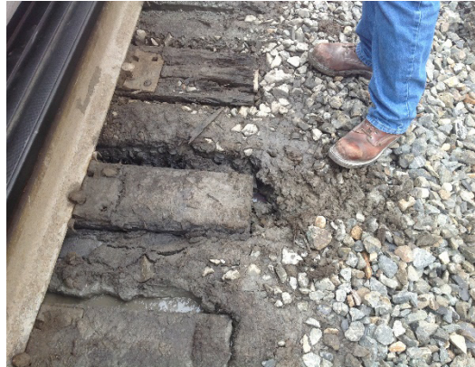
Figure 9. An example of timber rail ties under muddy conditions and experiencing weathering.
