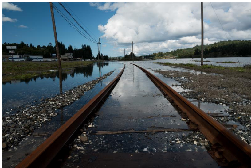
Figure 12. Concrete rail ties submerged during a flash flood. Image credit: Adobe Stock.
