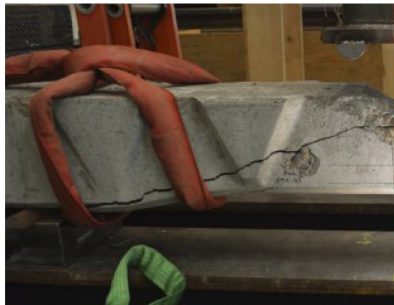
Figure 6. An example of cracking in a concrete rail tie.
