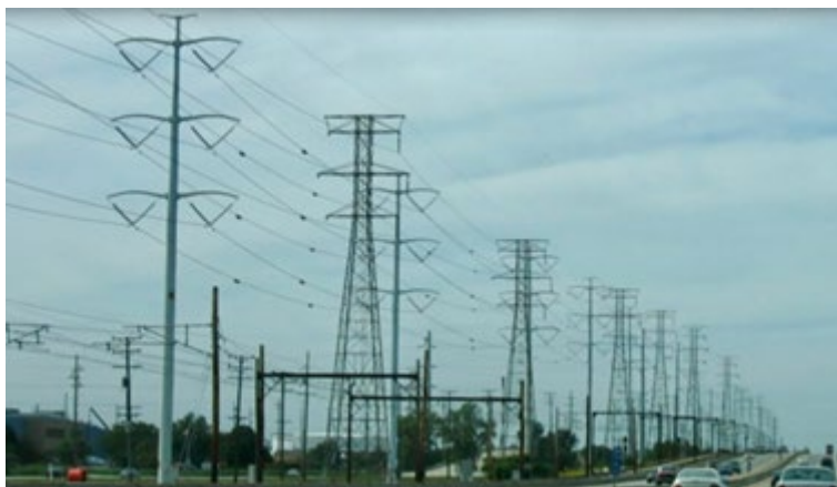
Figure 48. Longitudinal Transmission Line Along the Chicago South Shore and South Bend Railroad Parallel to the Indiana Toll Road
