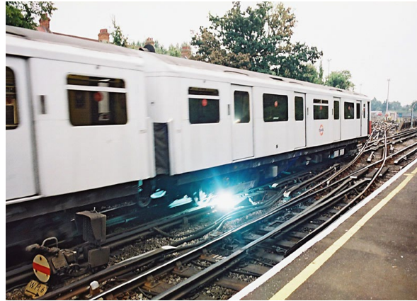
Figure 17. Visible Arcing Between the Lead Rail Vehicle’s Shoe and One of the Energized Rails on the London Underground (SPSmiler, 2005)
