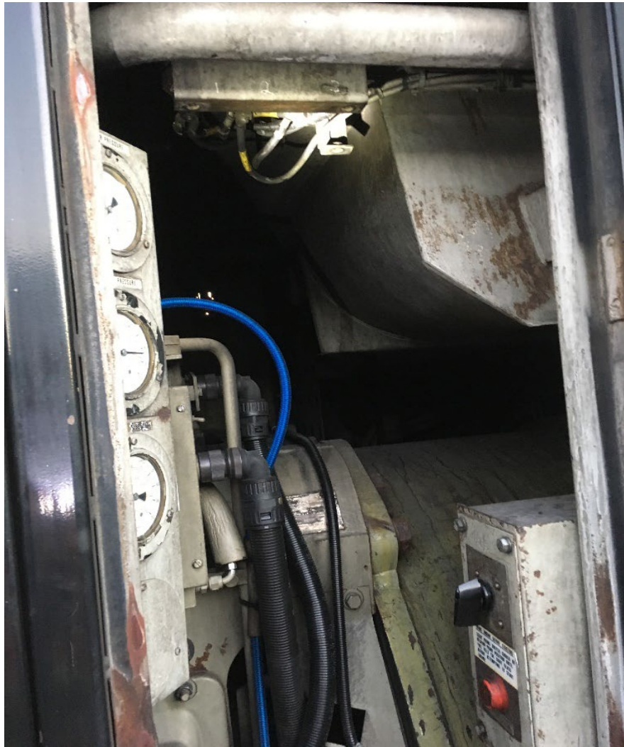
Figure 1: Missing high voltage electrical cover on GE locomotive; top of frame.
