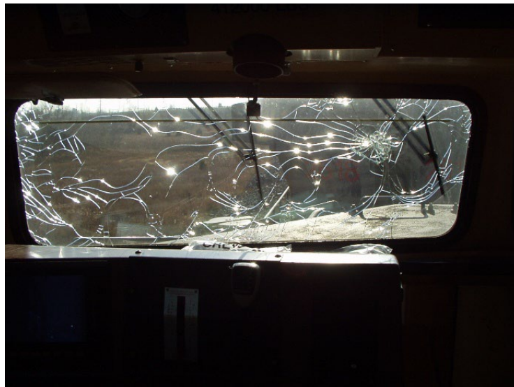
Figure 3: Failed Type I glazing
