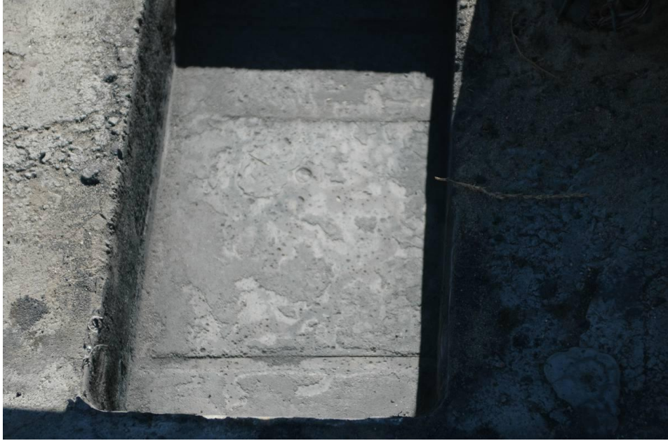
Figure A3. Cavity of Tie Number 190
