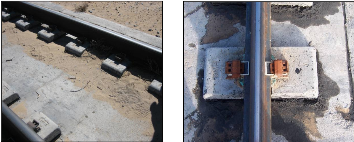
Figure 30. Fine Sand Deposit and Buildup of Gray Material around IDBT Tie Blocks
