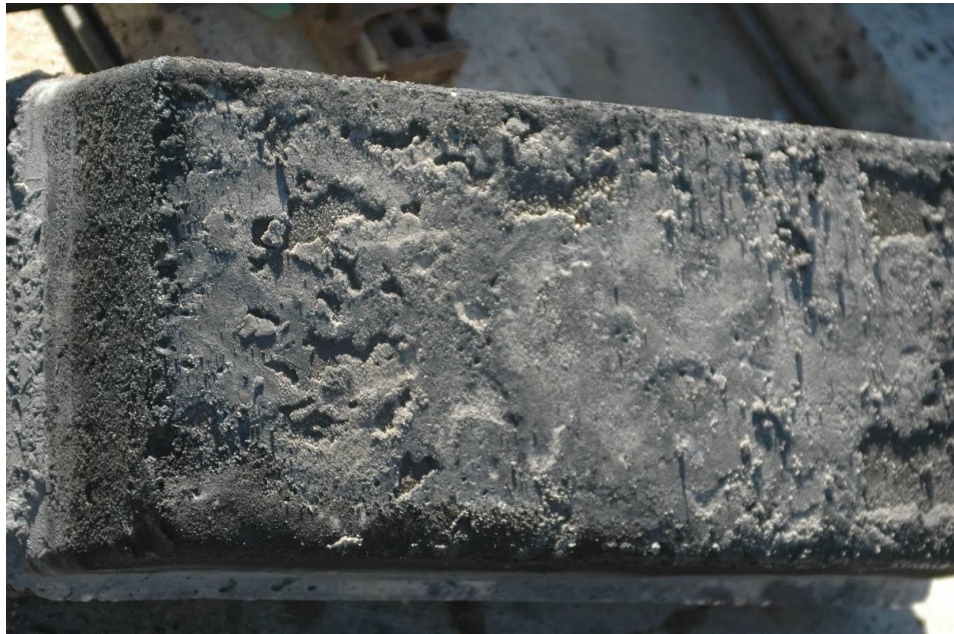
Figure A8. Bottom of Tie Number 151
