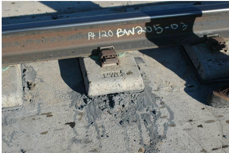
Figure A13. Tie Number 151, Showing Gray Material Discharged from Tie Cavity
