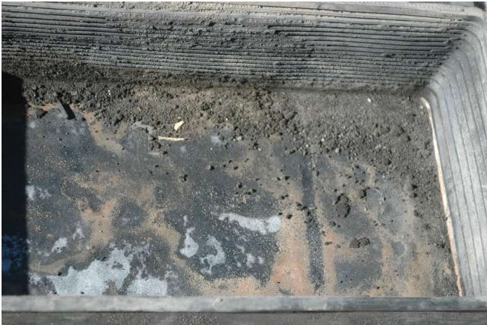
Figure A4. Inside of Boot for Tie Number 190
