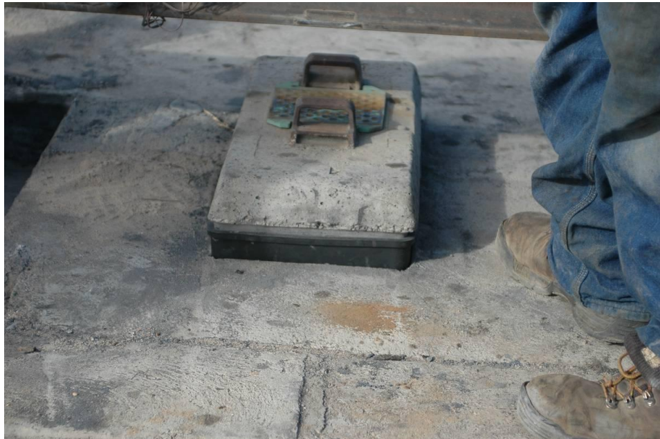
Figure A12. Tie Number 151, Placed Back into Cavity and Not Fully Seated
