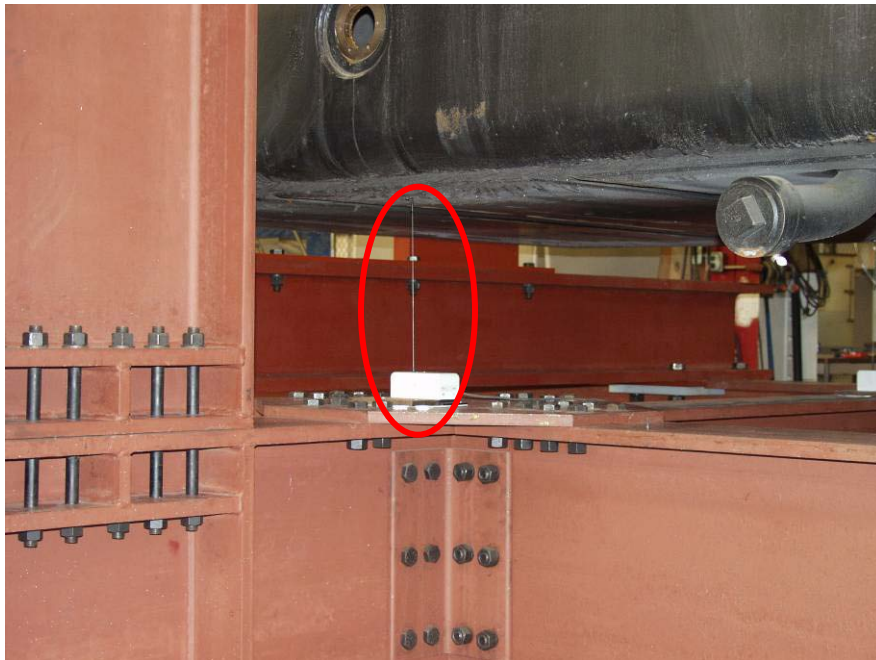
Figure 10. String Potentiometer Attachment to the Top Wall of Inverted Tank
