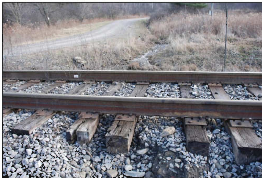
Uncontrolled drainage ran over the track and washed out ballast at this private crossing.
