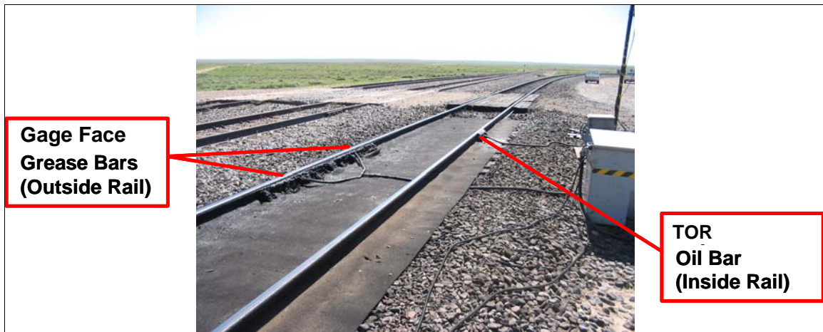
Figure 4. Lubrication Site in Section 26, with Gage Face Grease (High/Outside Rail) and TOR Oil (Low/Inside Rail) Applicator Bars Indicated
