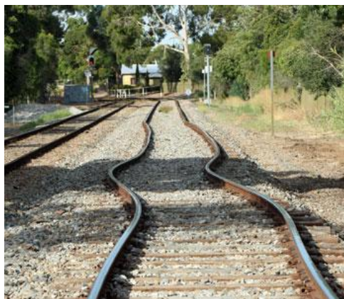
Figure 1. Buckling in a CWR
