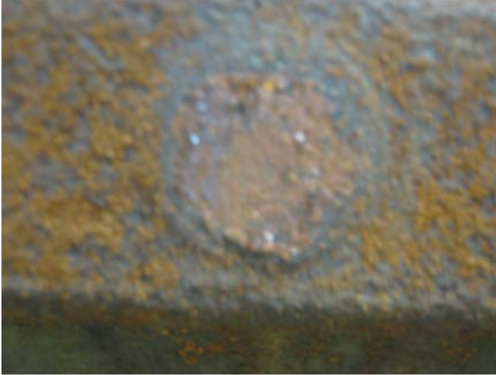
Figure 45. Low Quality IFW Joint due to Misalignment
