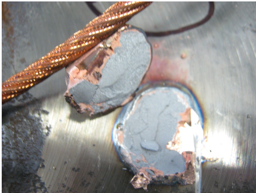
Figure 55. Fractured CAD Weld
