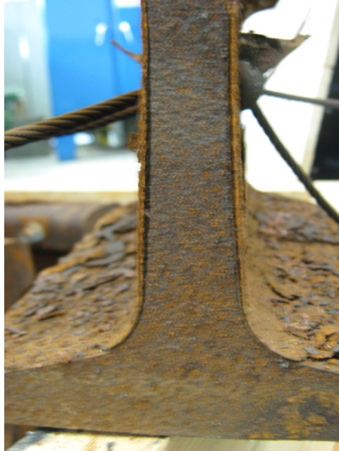
Figure 42. End View of Rail Showing Corrosion Products' Accumulation on Rail Web
