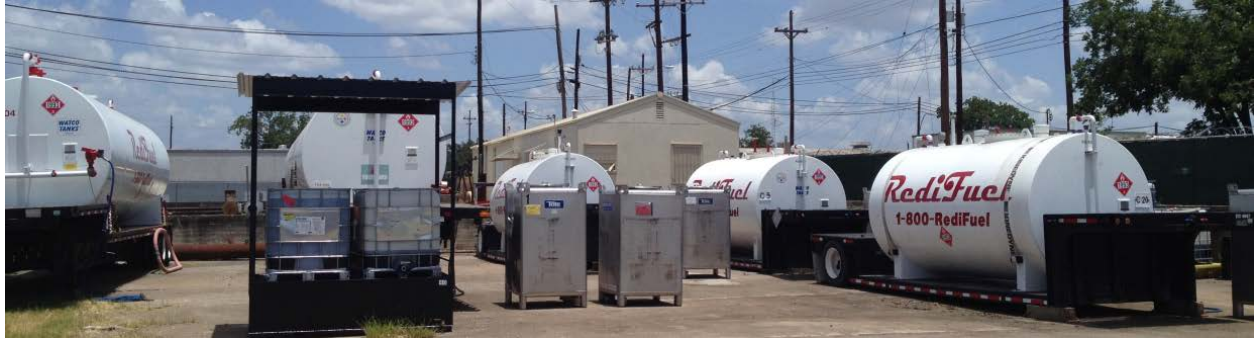
Figure 2. Fuel Storage Tanks and Fuel Totes
